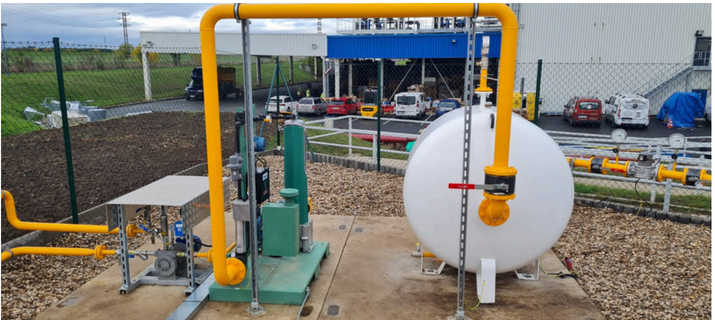
TXV supplying SNG to a factory
