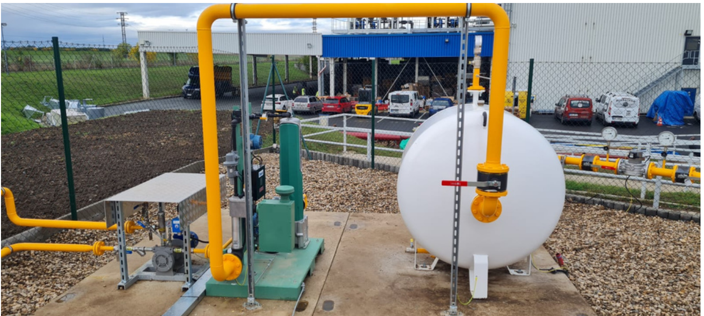
TXV supplying SNG to a factory
